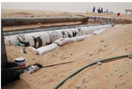
Damaged Bitumastic Tape Wrap System
