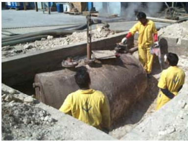
Equipment before SolarTech application
