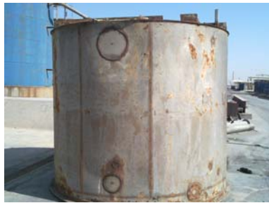
Damaged storage tank
